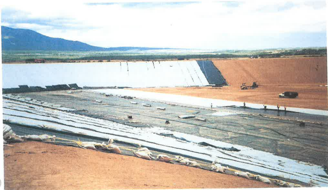
An installation crew deploys a secondary HDPE liner over a secondary GCL on the floor of the Monticello mixed-waste repository.
