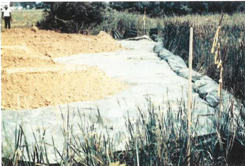
Photo 1. This swamp road is a classic example of a geotextile separation application.
