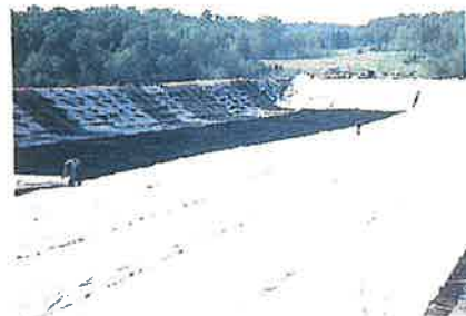
Photo 1. Geonet-composite drainage systems limit infiltration on the flatter slopes of landfill final covers.
