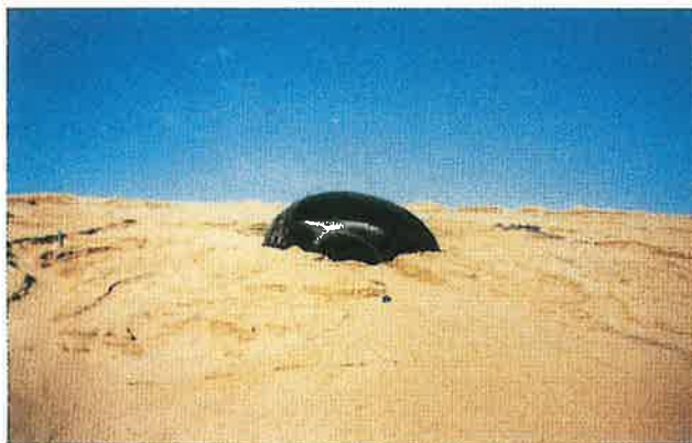
Photo 1. This small gas "whale" developed during the construction of a fairly standard final cover.
