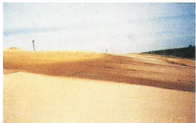
Photo 2. Failure on this slope occurred during placement of the pore pressure relief layer over the geomembrane. The sand and PVC geomembrane slid down the GCL.
