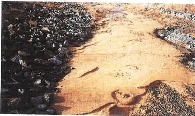
Photo 3. This very silty, fine-sand, vegetative-support layer is "flowing" from a landfill cover's side slopes.
