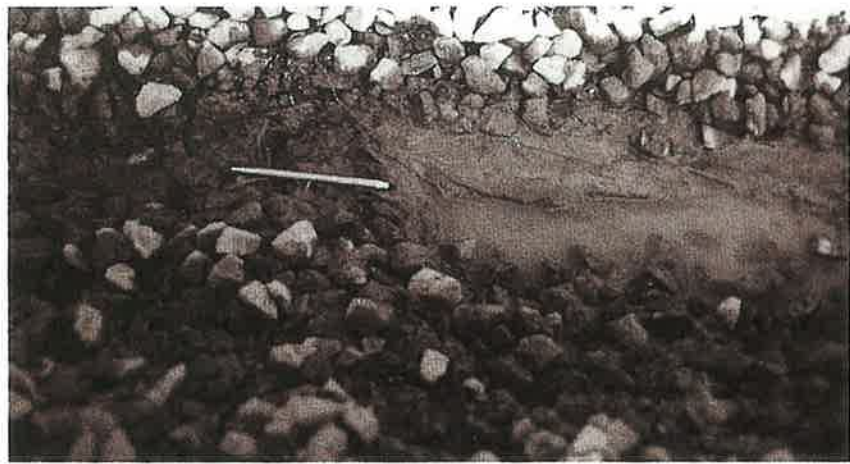
Photo 2. A geotextile was placed after rain filled the foundation excavation at this Greensboro, N.C. site. An excavation showed that water trapped beneath the geotextile was released only when the fabric ruptured.
