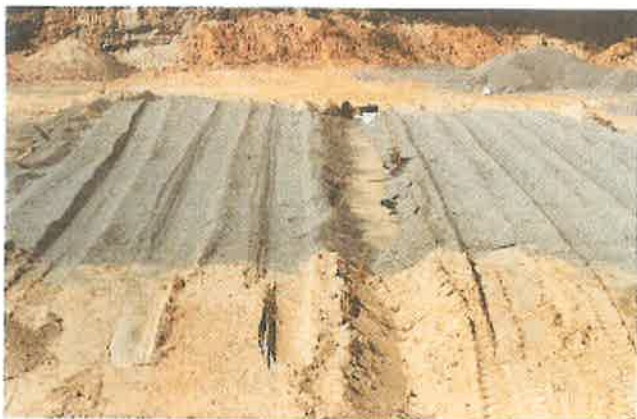
Photo 1. Well-defined ruts caused by a loaded dump truck mark the traffic lane.
