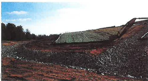
Photo 1. An ECB protects a 5H:1V slope at the Super Gro landfill, serving as a mulch while reducing erosion.
