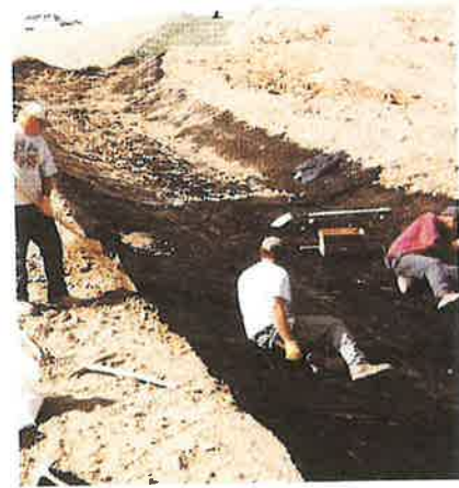
Photo 2. This three-dimensional geotextile, which lines a Pennsylvania-landfill down chute, saved more than $20,000 over riprap.
