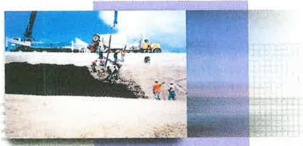
Geosynthetics Projects Category 2000 Award of Excellence Winner Presto Products Company, Appleton, Wis., and Colorado Lining International, Parker, Colo.
