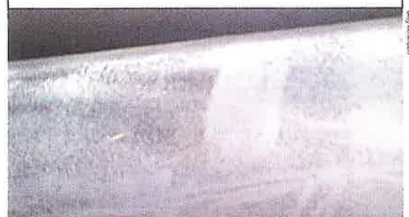
Photo 1: Geomembrane with inadequate spray-on texture bond.
