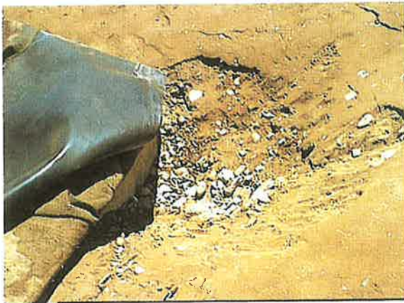
Photo 2: Scour of bedding layer is evident after geomembrane removal.
