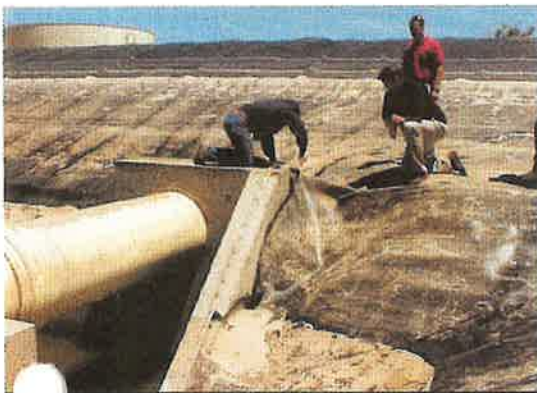
Photo 1: A significant length of geomembrane was pulled from the batten strip.
