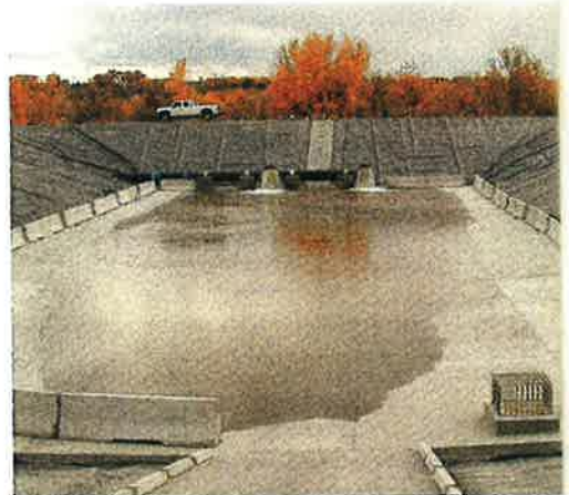
Photo 1. The completed access ramp and base clear the way for the geosynthetic redesign of the structure.
