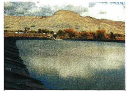
Photo 2. The rehabilitated reservoir is finally able to begin serving the water district.
