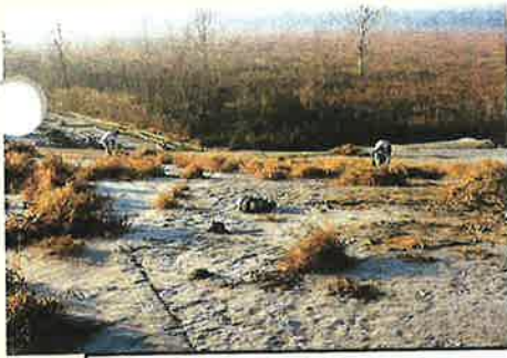
Photo 3. Invasive grass in exposed geotextile.
