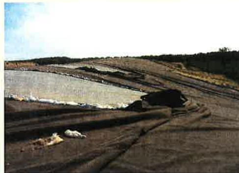
Photo 2. UV degradation of drainage composite.
